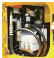
Fuel Feed Pump
